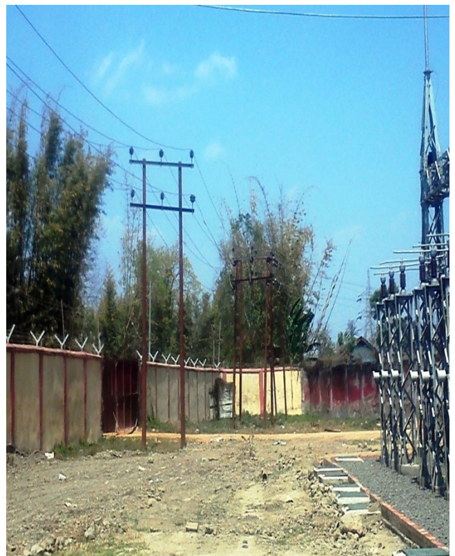
33 kV (H Pole) line inside substation
